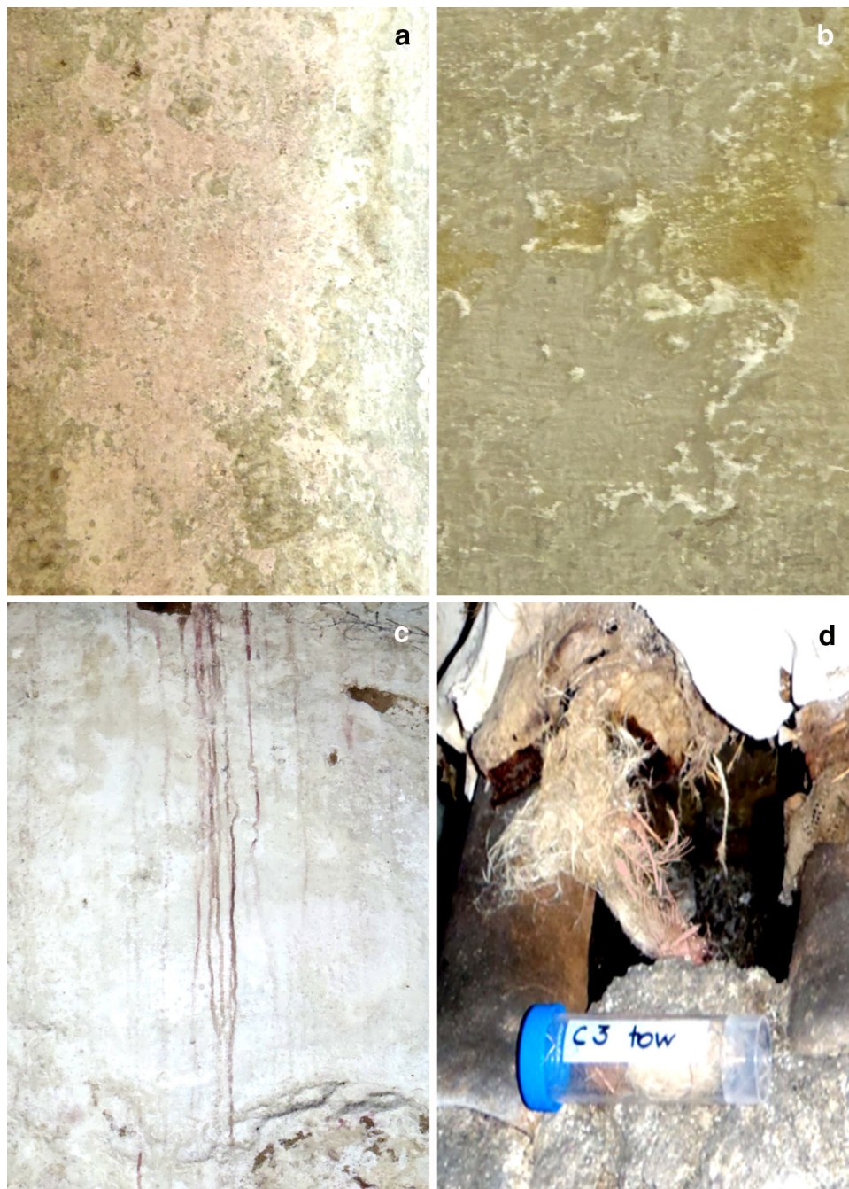
Fig. 3 a Sample W1: rosy discolored wall. b Sample W2: salt efflorescence with yellowish discoloration. c Sample PS: wall showing purple stains. d Sample C3: stuffing material, showing orange to rosy discoloration (pictures: Sterflinger)
