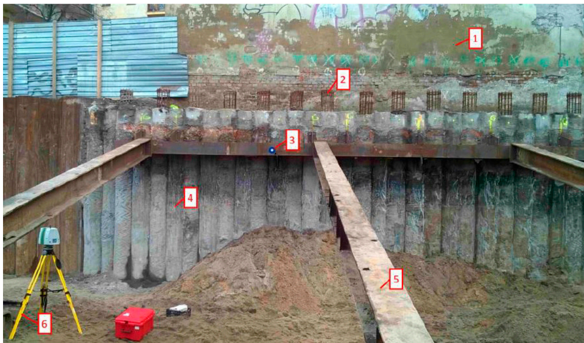
Figure 1. Protection of deep excavation by means of continuous flight auger (CFA) palisade: (1) the wall of the nearest existing building; (2) reinforcement cage; (3) special target used as the tie point for combining scanner positions; (4) palisade made of CFA piles; (5) steel strut; and (6) position of the laser scanner.
