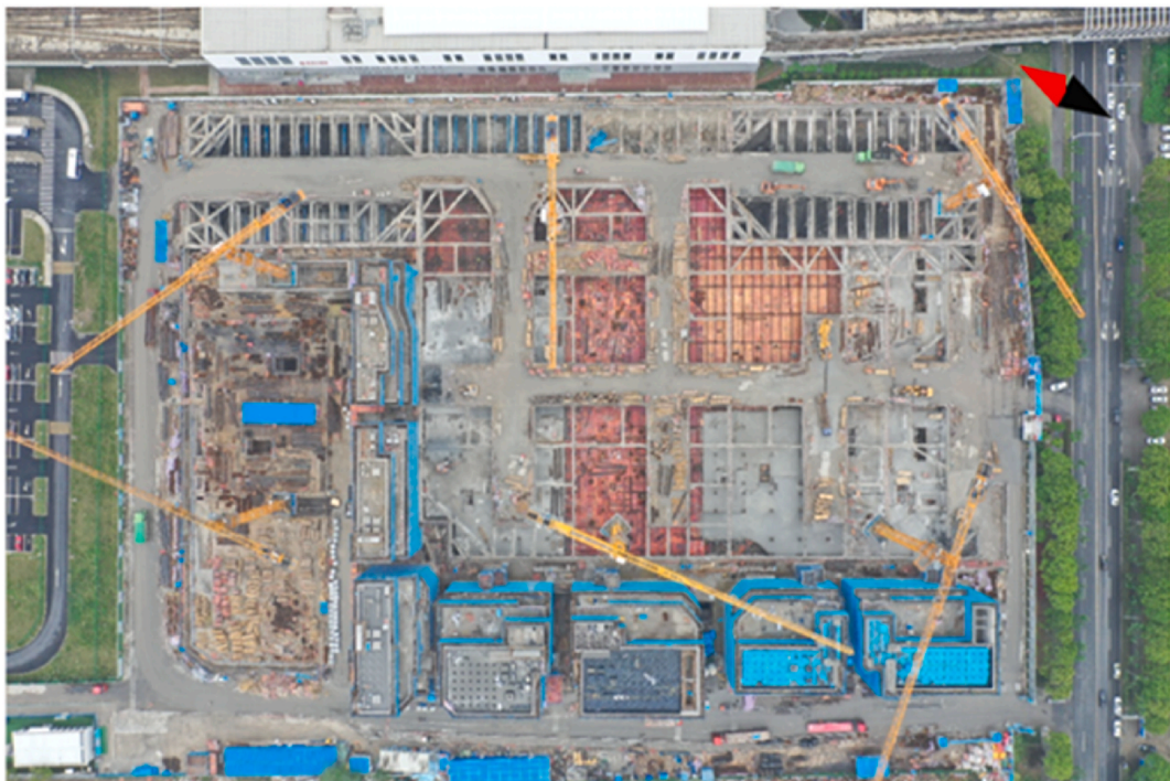
Fig. 5. Aerial photo of 07F-01 regional parcel project, in the Unit 19, Nanqiao New Town, Fengxian District ( Drone footage ) .
