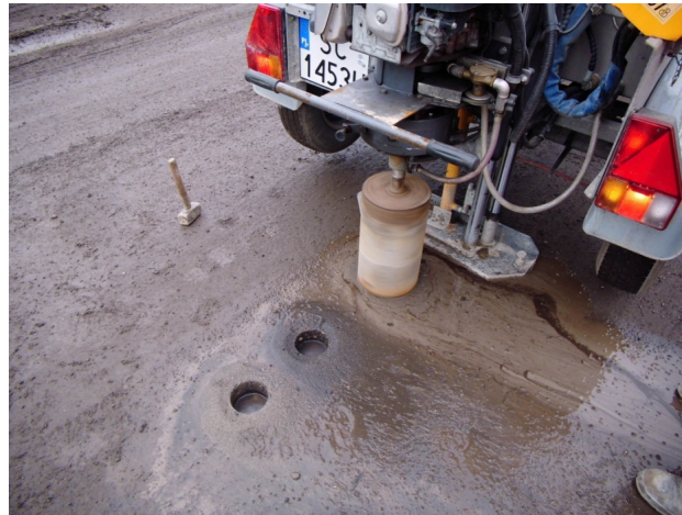
Figure 7. The drilling of the samples from the tested trial road pavement (AM-100%).
