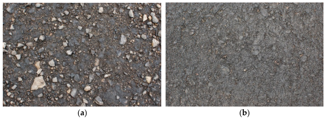
Figure 8. Trial road sections: (a) “gravel”—cold rolled destroyed asphalt material and (b) hot, recycled in 120 °C, RAP of the same material.
