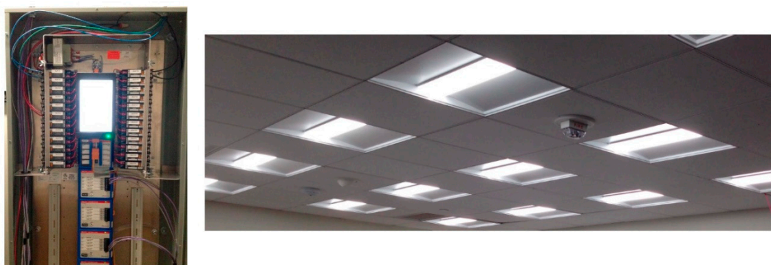
Figure 3. Photo of the lighting system controller (left) and lighting luminaires (right).
