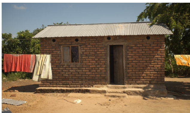
Figure 5. Front view of house B after installation of the eave tubes. The bedroom is on the left.
