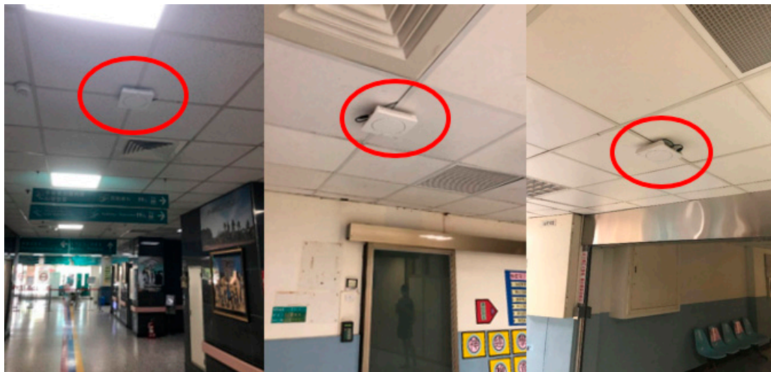
Figure 14. The installation of Lbeacons in the outpatient area of NTUH-Yunlin.
