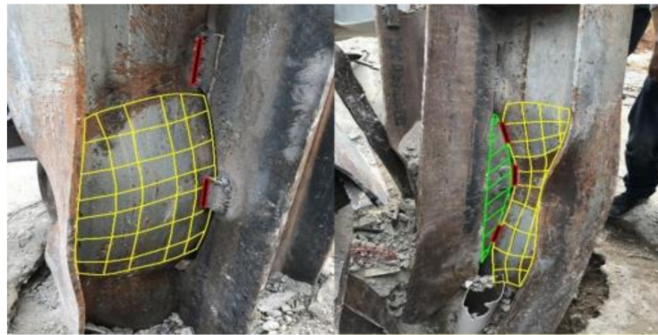
Figure 5. Buckling deformation and welding of C6 steel column. From the Investigation Report on the Collapse of Xinjia Hotel, Quanzhou City, Fujian Province.
