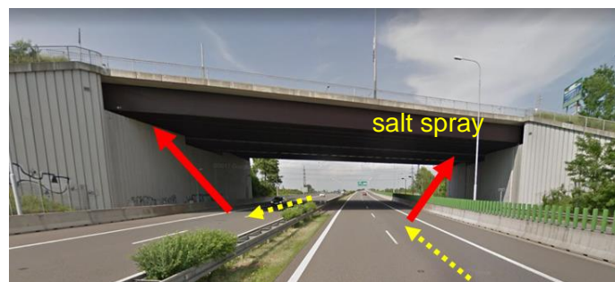
Figure 1. Tunnel-like conditions under the bridge (road bridge over highway D1 in the city of Ostrava, Czech Republic).
