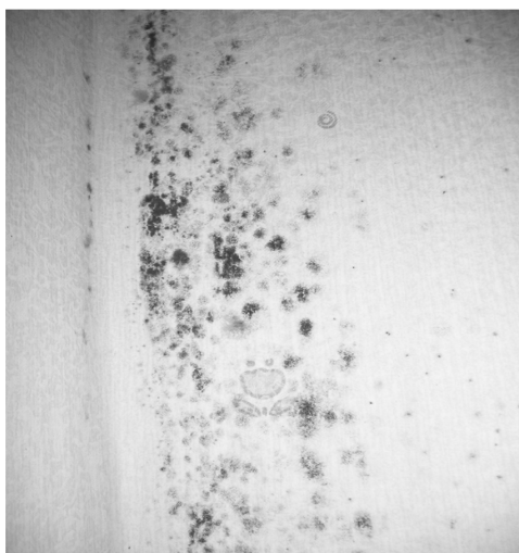
Fig. 2. Fungal growth on apartment wallpaper with continuous humidifier use. The condition of wall paper was photographed during 15 day of humidifier operation.
