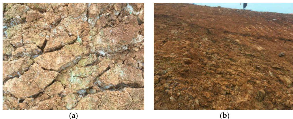
Figure 2. Disintegration damage under the action of wet and dry cycles: (a) disintegration damage; and (b) severe soil damage.
