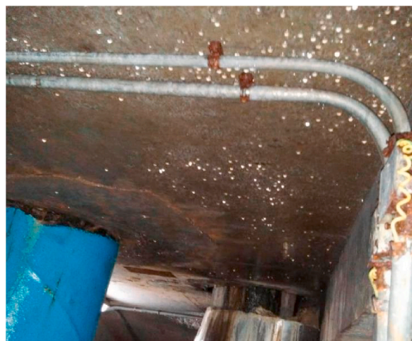
Fig. 3. Condensation phenomenon inside utility tunnels in summer.
