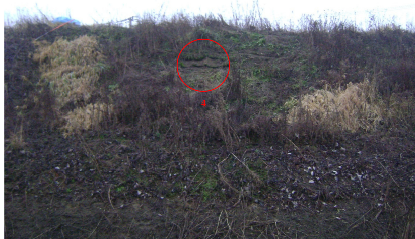
Figure 3. Closer view of location 4 of the protected slope in Nieboczowy (state of slope on 18 January 2020). In the circle: exposed recycled natural and synthetic fibers (RNSF ropes); to the right of the circle: wool rope.
