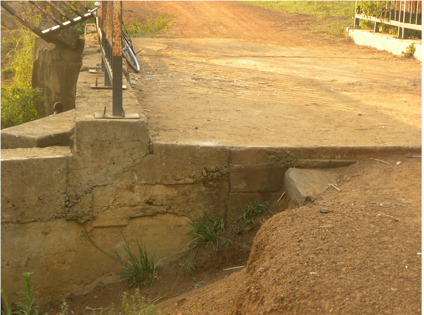
Fig 3. An example of deteriorating infrastructure. In this example, the respondent detailed numerous accidents that have occurred due to this degraded bridge on a busy road.
