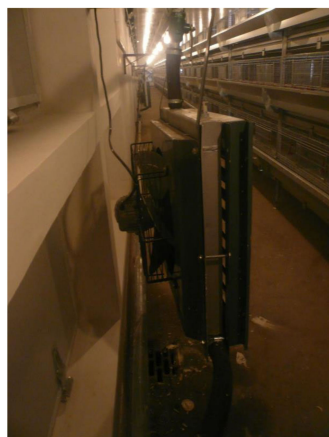
Figure 5. A small fan was installed at the back of the radiator.
