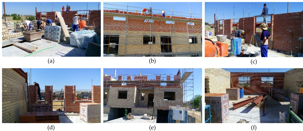
Figure 5. Different moments of the work unit in the case study: construction of an exposed brick façade: (a) Site Organisation; (b) Work on Scaffolding; (c) Personal Protection; (d–f) Fall Risks.
