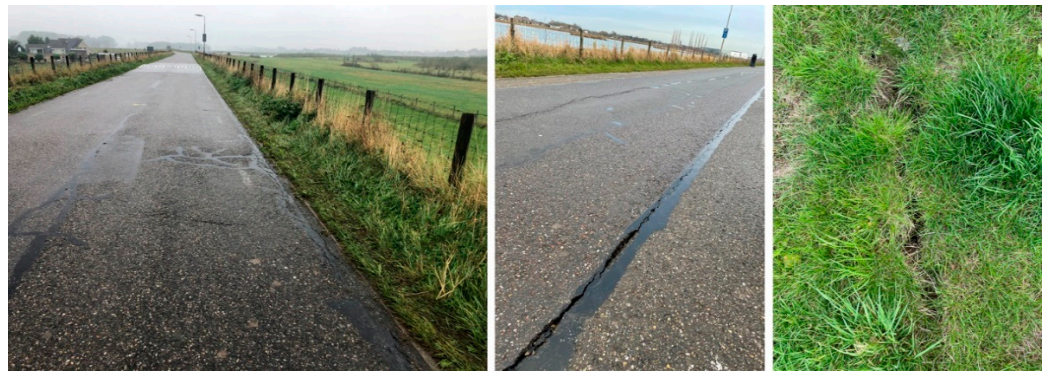
Figure 8. Presence of cracks on the embankment road and slopes.
