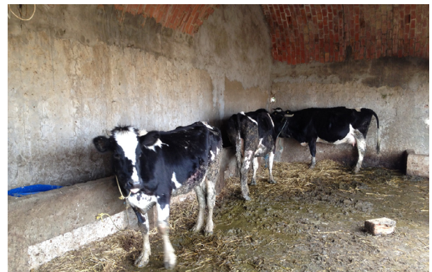
Figure 5. Cattle shed where the Hyalomma scupense tick is usually present; note that the walls are not roughcast, with several cracks and crevices.
