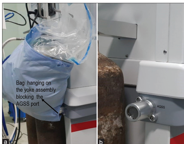
Figure 1: (a) Bag hanging on the yoke assembly blocking the anaesthesia gas scavenging system (AGSS) port, (b) AGSS port after the bag was removed
