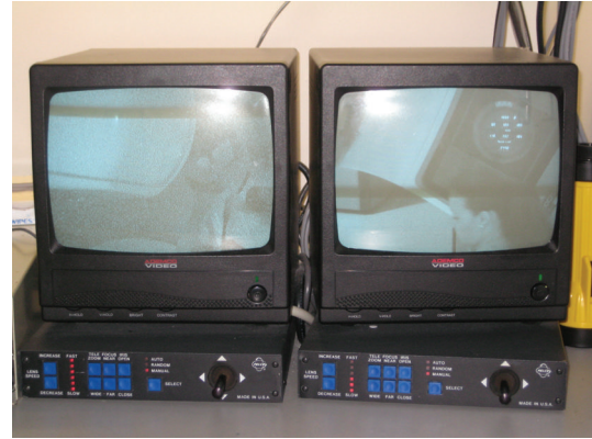
FIGURE 7: A remote monitor bank.
