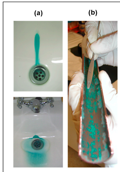
Figure 1. The effect of microbial biofilm formed on copper pipes household system: (a) bluish green stains in two sinks; and (b) two-year-old pipe affected by MIC.
