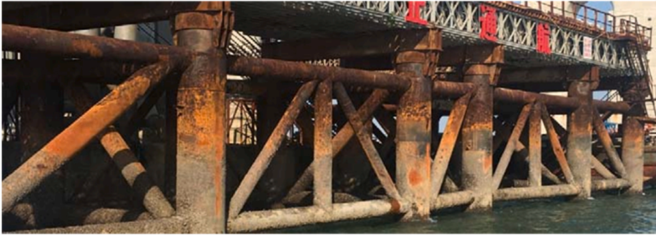
Fig. 2. Corrosion status of the steel construction wharf after 4 years of operation.
