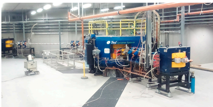
Figure 2. The new high-energy (70 MeV) and high-current (750 \mu\text{A} ) proton-beam cyclotron installed at LNL-INFN (Legnaro). One of the two main switching magnets may be seen on the right.
