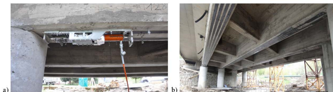
Figure 16. Strengthening of the bridge in Komańcza, republished from [11]: (a) prestressing the CFRP strip; (b) view of the bridge after strengthening.
