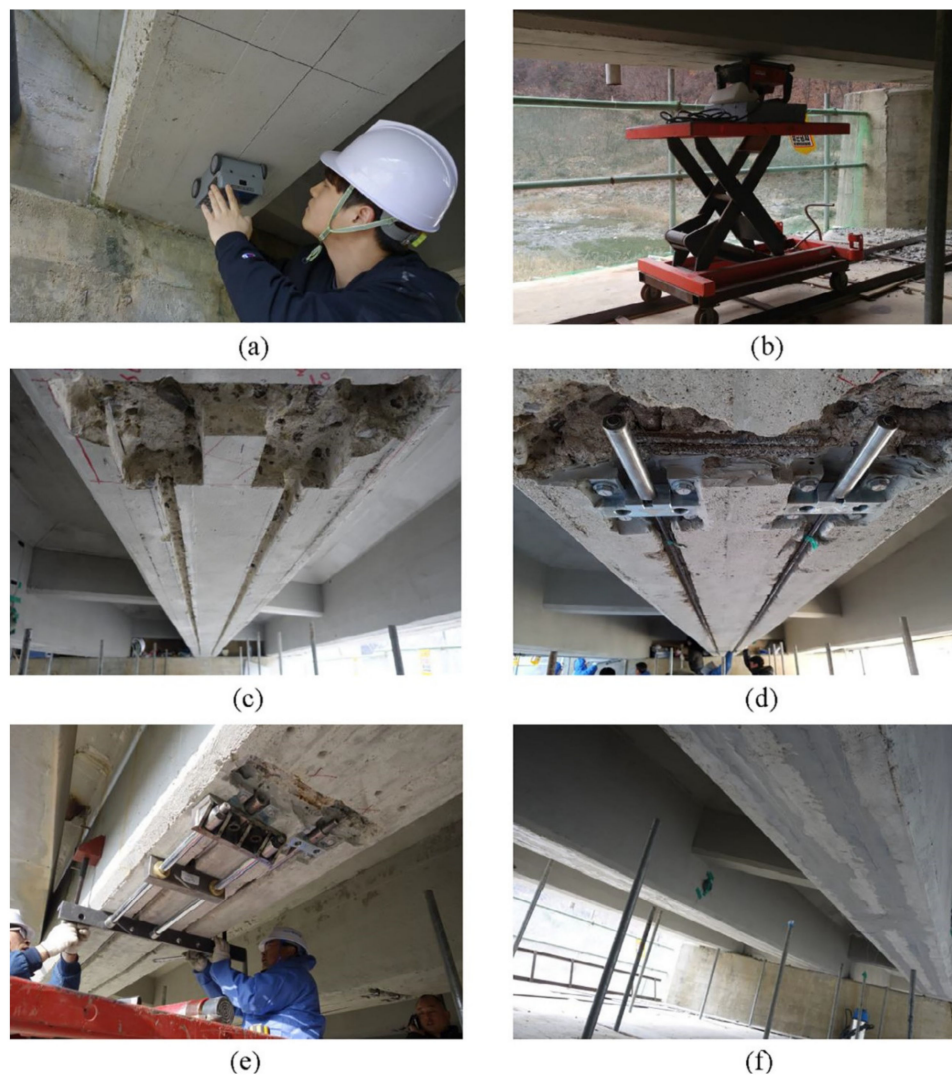
Figure 17. Process of bridge strengthening: (a) inspection to identify the thickness of the covering and the location of the steel reinforcement; (b) cutting the grooves; (c) view of the grooves; (d) installation of the anchorage and the CFRP bars.; (e) applying prestressing; (f) filling the grooves with an epoxy. Reprinted with permission from ref. [143]. Copyright 2018 Elsevier.
