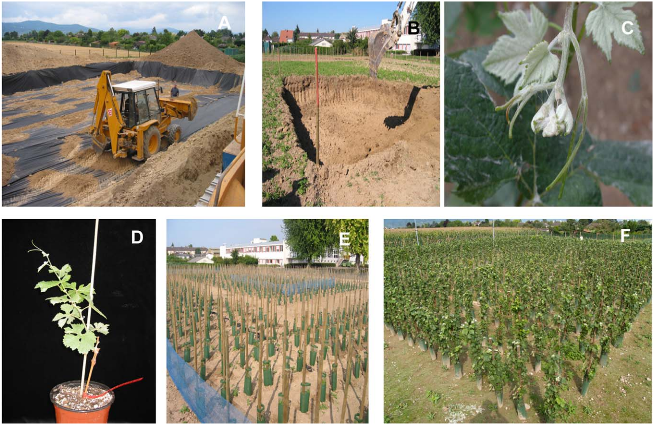
Figure 2. Construction of the experimental site and initiation of the trial in Colmar. (A) Laying of the microporous geotextile membrane. (B) After filling with soil from the site, preparation of the area that will receive soil from the GFLV-affected vineyard. (C) Leaves of the Pinot Meunier variety. (D) Pinot Meunier plant (leaves and stem) grafted on a GM rootstock (trunk). (E-F) The trial after planting in September 2005 and in 2008, respectively. doi:10.1371/journal.pbio.1000551.g002
