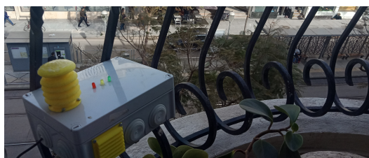
Figure 4. Nomadic sensor node installation.
