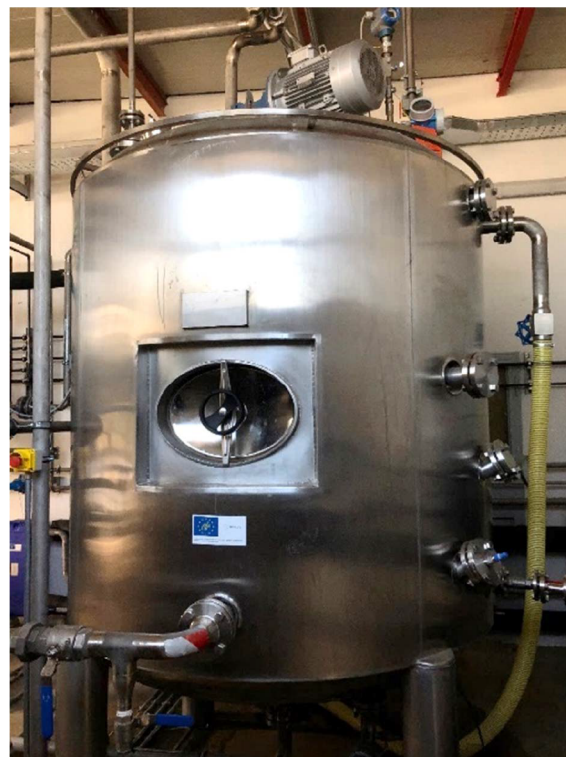
Figure 1. Bioreactor located at the MEWLIFE plant in the NextChem site in Rome.
