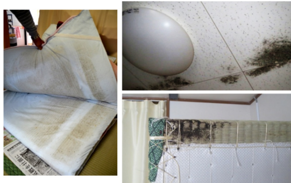
Figure 3. Fungal contamination in temporary housings.
