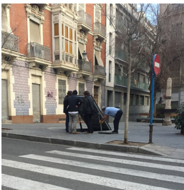
Figure 9. Image showing the opening of the hydraulic access to the Plaza Balmis refuge on Canalejas Street. This entry is being modified by a fixed type for greater security.
