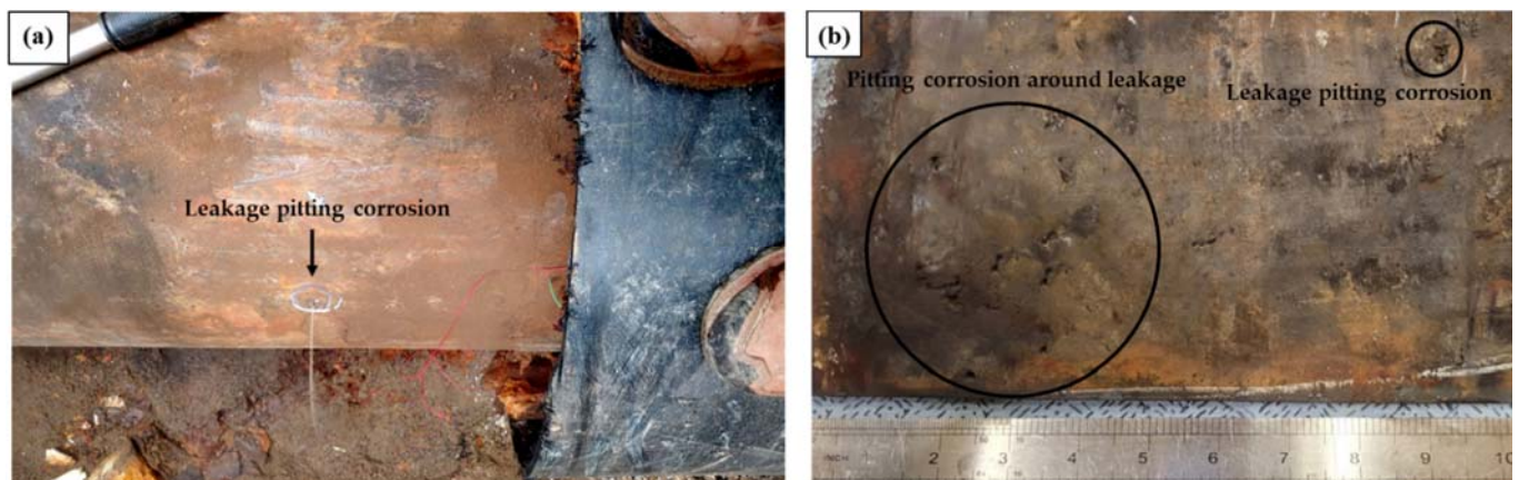
Figure 2. Photographs of the failed pipe: (a) water leakage resulting from pitting in the failed pipe, (b) external surface of the failed pipe around the leakage area.
