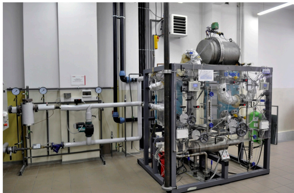
Figure 6. Picture of the ORC power plant.
