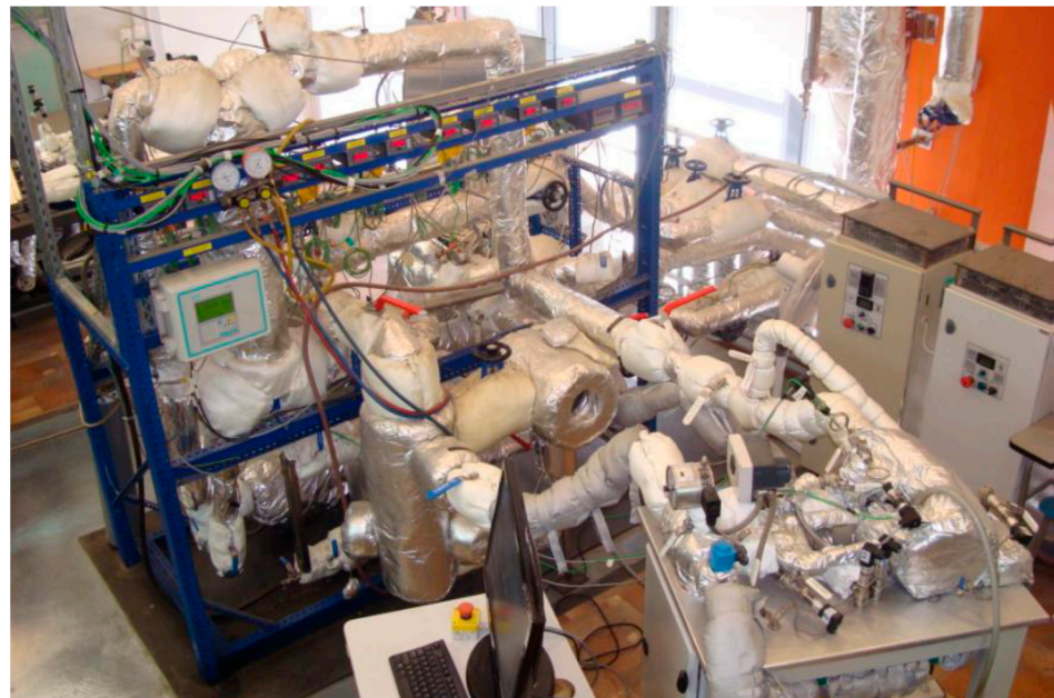
Figure 4. View of the experimental ORC power plant at IMP PAN.
