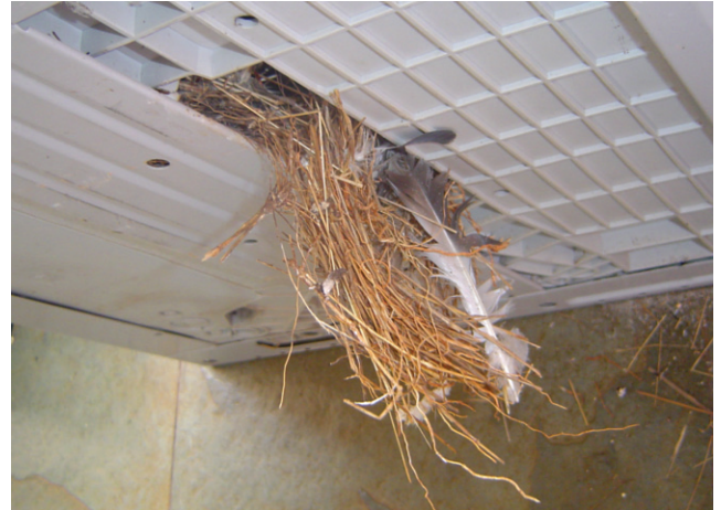
FIGURE 4: Panel D. Empty pigeon nest inside the air-conditioning unit. An empty nest full of avian mites was found inside the air-conditioning unit
