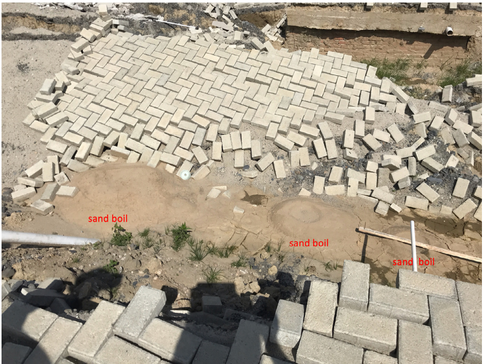
Fig. 2. Example of three cone-shaped sand boils indicating soil liquefaction.
