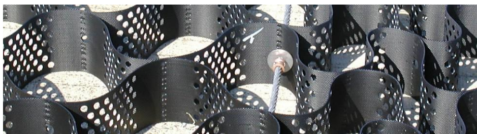
Figure 7. Photo showing typical installed copper stop sleeve/stainless steel washer bearing assembly inside an empty geocell.
