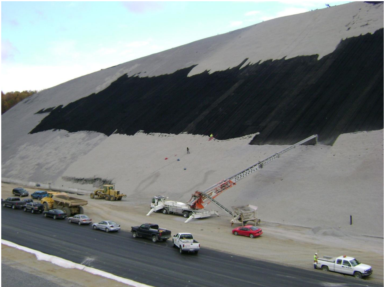
Figure 11. Photo showing stone aggregate infill in progress on the Large Cut Face.
