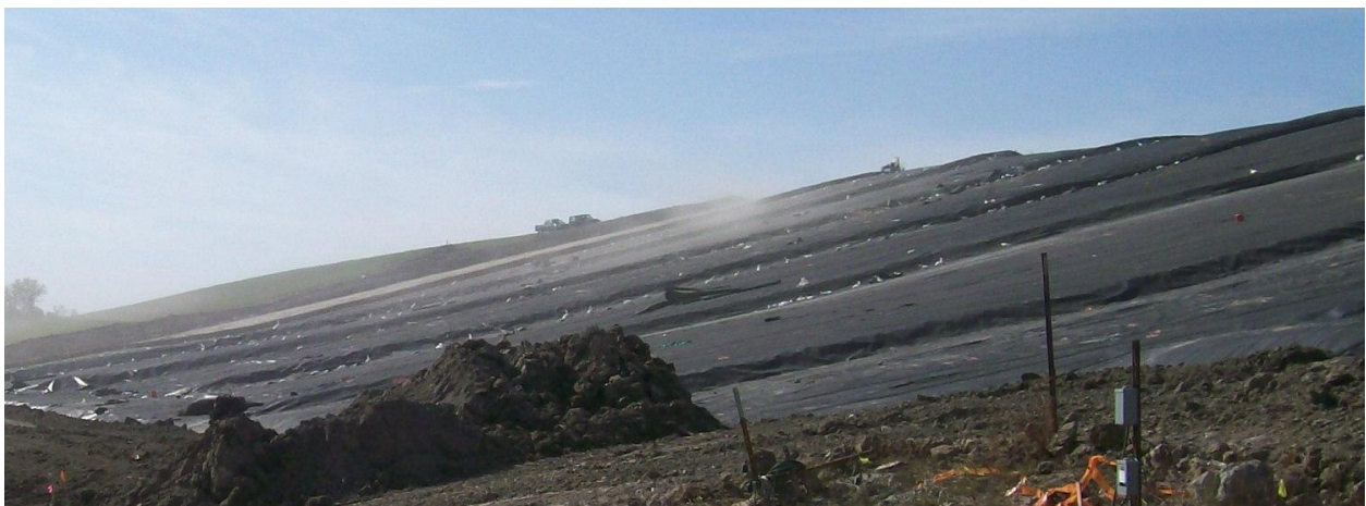
Figure 1. Photo of 1.0-mm thick HDPE exposed geomembrane cover. Soil windrows capped with geomembrane are visible in shadowed relief on the slope face.
