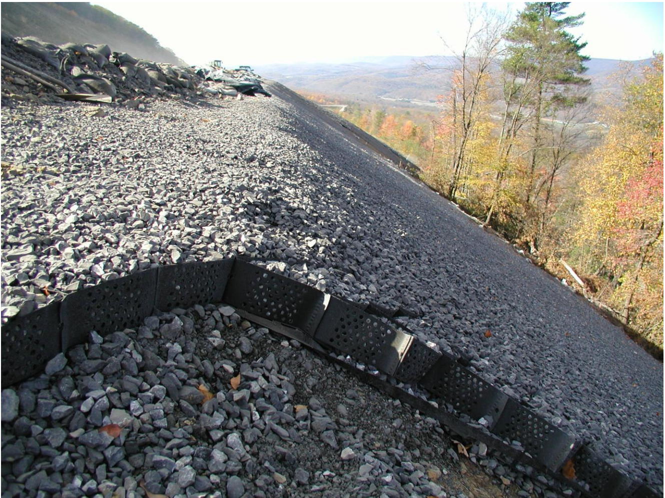
Figure 5. Stone aggregate-filled geocell overlying a geogrid layer. The slope shown varies in inclination from 1H:1V to 1.5H:1V.
