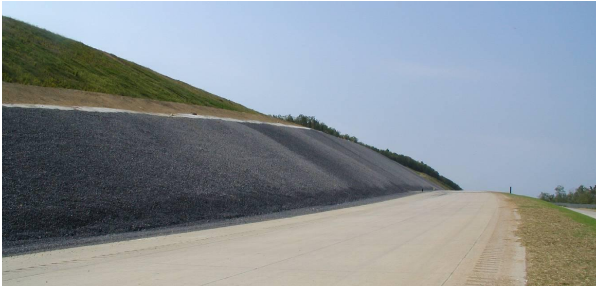
Figure 12. Photo showing appearance of a section of armored slope cover following aggregate infill.
