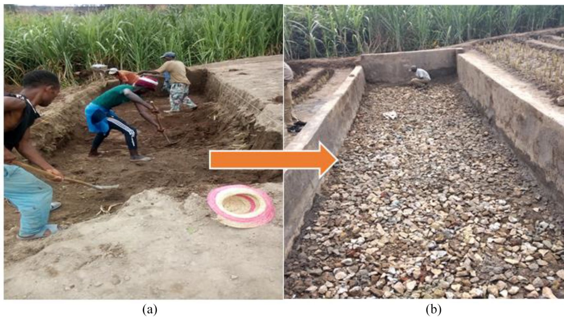
Figure 6. Construction of open space between 2 wetlands: (a) during excavation and (b) after construction.
