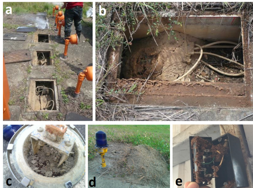
Figure 4. RIFA destruction to electric facilities in Taiwan. (a,b). RIFA colonized in cable boxes in Taoyuan International Airport. (c,d). RIFA invaded into a runway lamp (c) and a colony located beside a runway lamp (d) at Songshan Airport. (e). RIFA invaded a circuit breaker in a resident's house.
