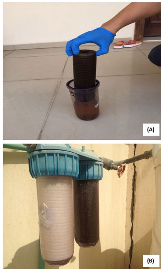
Figure 3. (A) Filter membrane showing heavy accumulation of residues; the beaker shows the brownish slurry within the POU unit. (B) Comparison of new filter (left) and one that had been installed for four months (right). The cartridge taken out of the filter is shown separately on the right.
