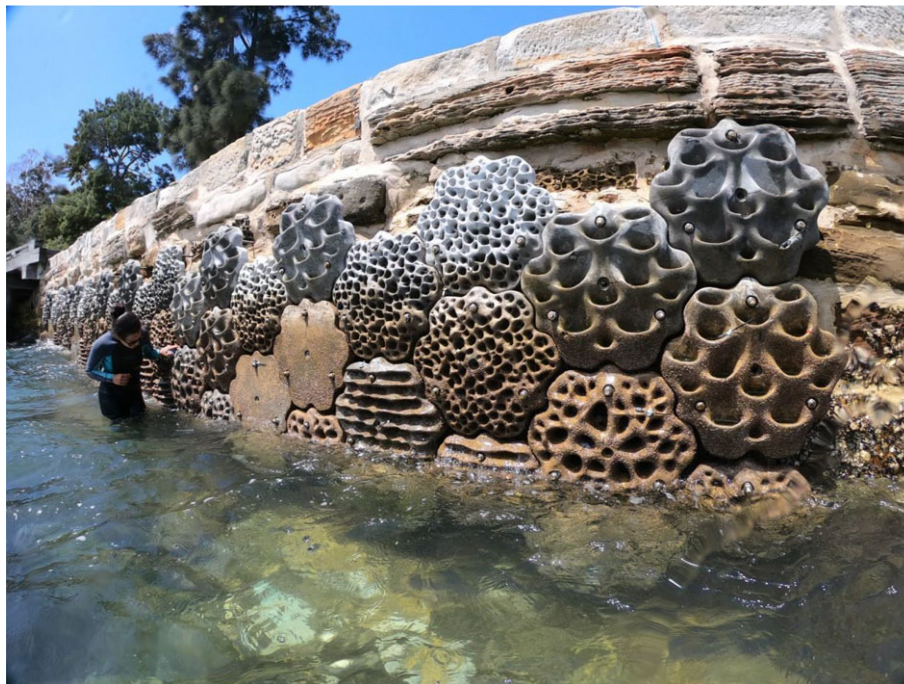
Figure 2. The Eco-engineered site, approximately 6 months following panel installation (photo credit: Alex Goad). (Online version in colour.)
