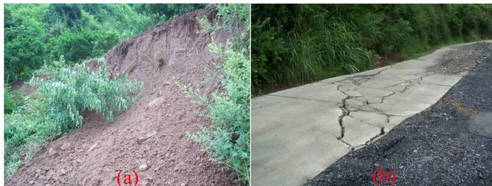
Figure 3. Deformation characteristics of Shuping landslide (photographs taken by Yuanyao Li).
