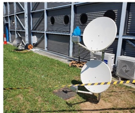
Figure 15. B-LiFE deployment in Turin, Italy, during the COVID-19 crisis: installation of 2 Eutelsat SatCom dishes.
