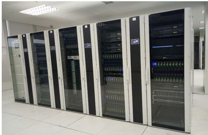
Figure S3 Part of supercomputing platform.
