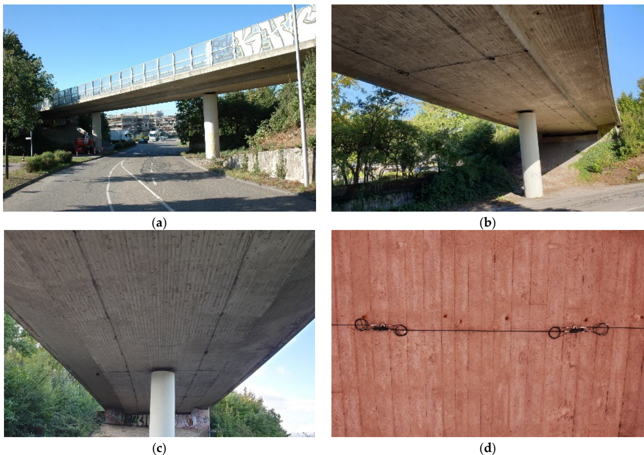
Figure 4. Overview of the bridge and the monitoring system: (a) Overview of the bridge; (b) view of installed sensors; (c) sensor distribution; (d) an LGFBG sensor with 2.05 m gauge.
