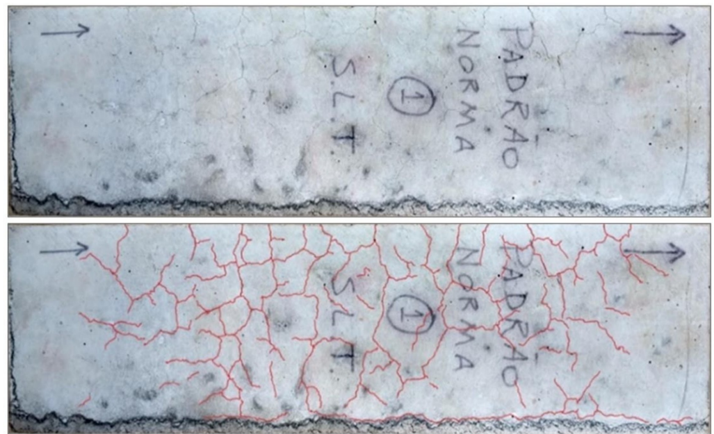
Figure 10. Typical mapped fissures (TOP— real images; BOTTOM— highlighted in red) on a face of the STL0 St prism.
