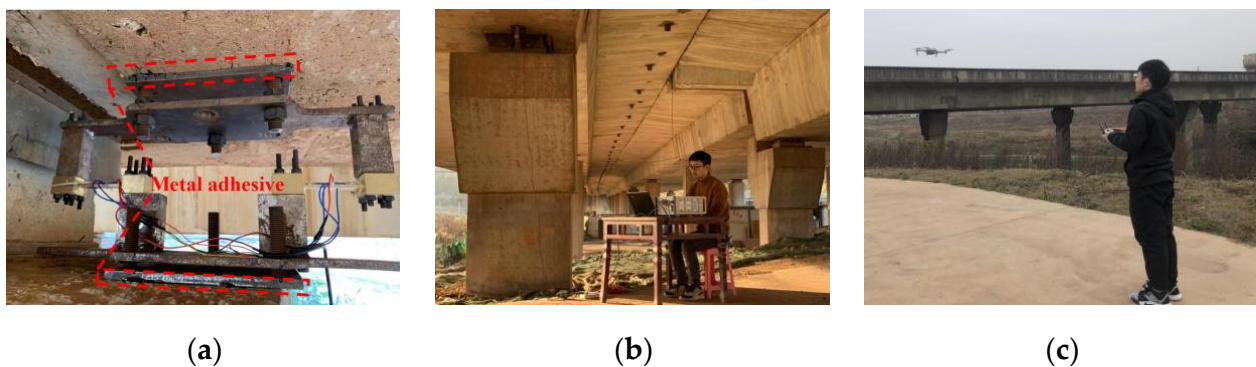
Figure 13. On-site installation of BRT-1 rotation monitoring device (a) device installation; (b) overall setup; (c) UAV photography.
