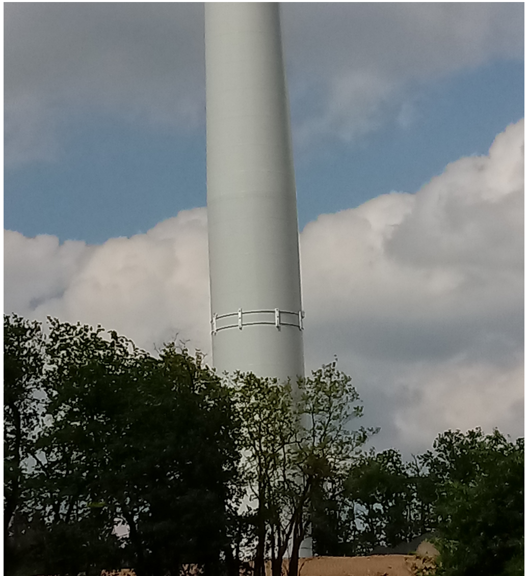
Figure 19. The system prototype mounted on a wind turbine at the test field. The system consists of eight Detection modules fixed on the tower wall and the Decision-making system placed inside the tower.
