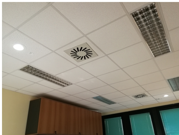
Figure 5. Ceiling: LED lamps, IR sensors, and neon lights.
