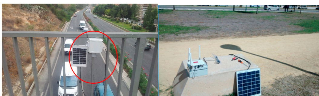
Figure 16. Different installations for UIS nodes. (a) UIS ULT node installation; (b) UIS Receiver node with solar kit.
