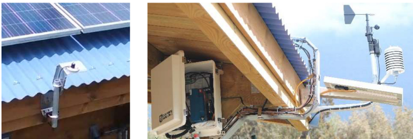
Fig. 5. Meteorological sensors and systems (a pyranometer on the left, the anemometer and the data logger on the right).
