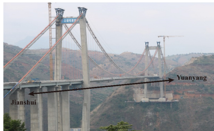
(b) Photo of Honghe Bridge project
