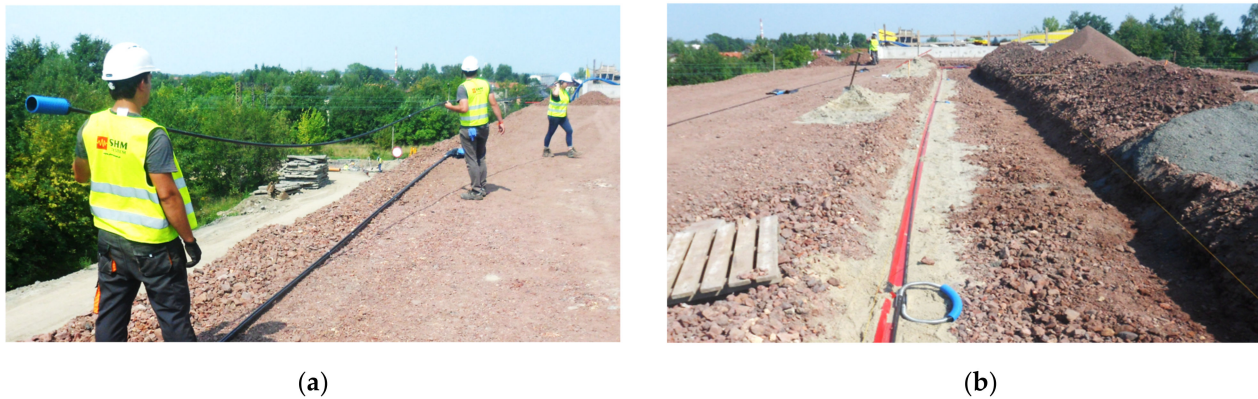
Figure 22. (a) The view of 3DSensor just before installation in the embankment; (b) the view of ready measurement line with 3DSensor and inclinometer casing.
